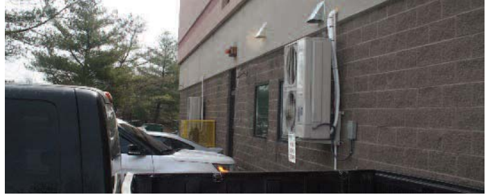
The VRF system consists of two five-ton heat pumps supplying conditioned air to the showroom/office space.
