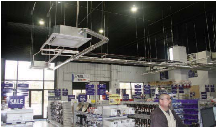
D-STRAT™ fans were used in showroom/office area to direct heated air down from 20-foot ceiling.
